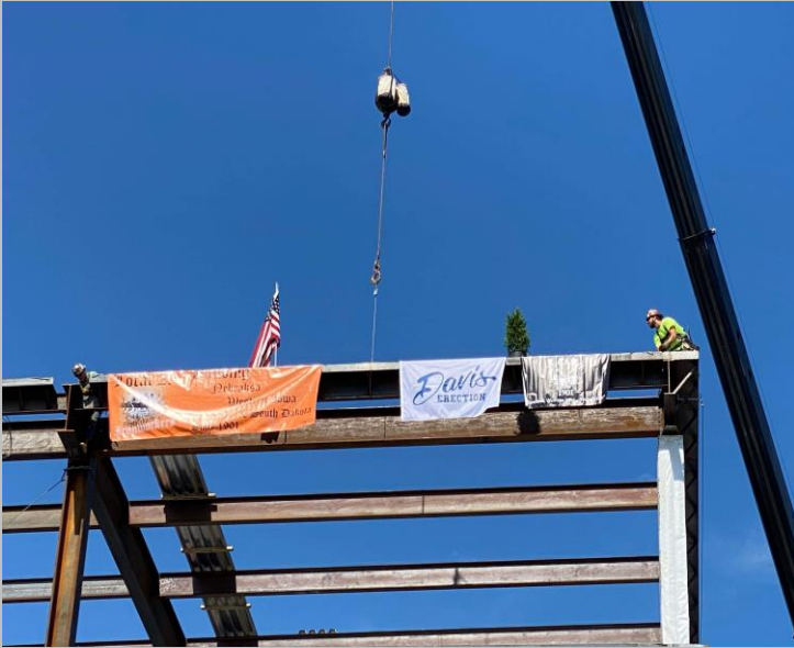
Tyler Seals and Layne Pofahl connecting the top out beam on Mike Fahey Complex
