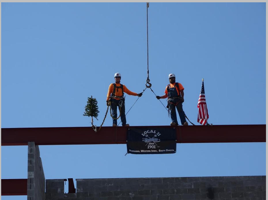
Jason Fox Jr. and Jonathan Retchless connecting the top out beam on SCC Technology Center
