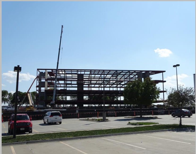
Mitch Brazina, Jason Hunt, and Joe Tyson installing deck at SCC Technology Center
